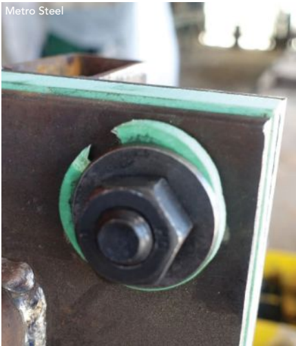
Fig. 5. Thermal washer failure at bolt with regular oversized washer.
