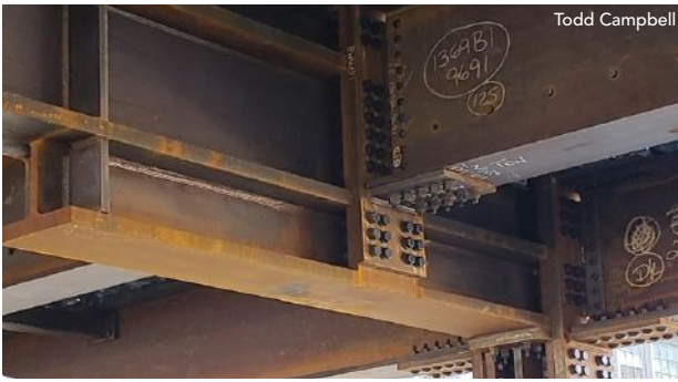
Fig. 4: A complex yet constructable transfer girder detail where the girder steps down.
